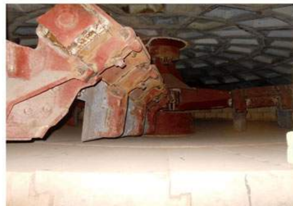
炉内件 Furnace inner parts
